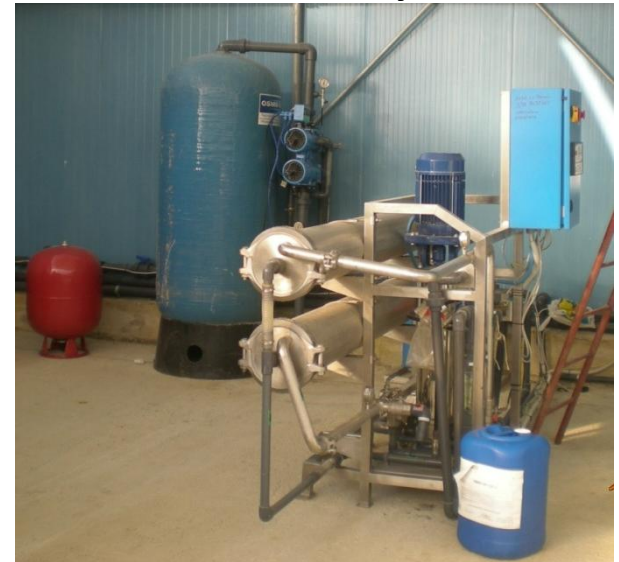
Reverse osmosis system
